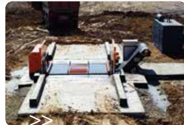
Connection power and water filling
